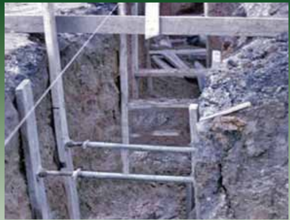
Simplex SE Series Trench Braces are used to shore up the walls of this trench for the repair work of underground water pipes.
