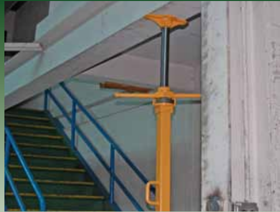
This RS Series Roof Support was used to support a horizontal I-Beam while weld work was being done on the verticle I-Beam.
